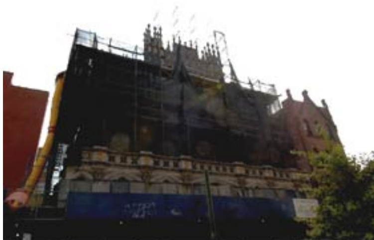
Harlem's dazzling St. Thomas the Apostle is shrouded in preparation for demolition.
